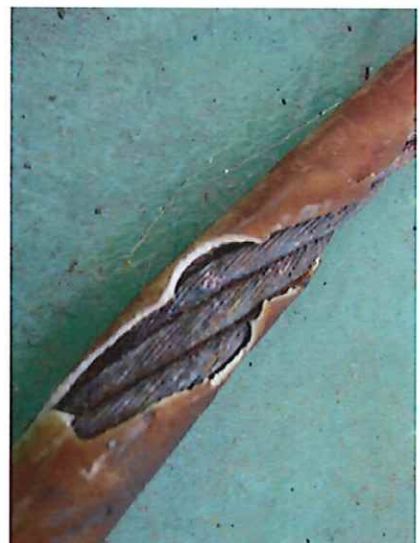
Figure 2. Corrosion beneath plastic sheathing.
