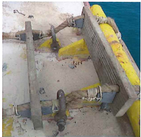
Figure 2. Pilot ladder incorrectly secured to the deck using D-shackles to choke the side ropes.
